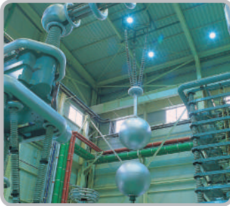
High Voltage Test / Impulse Test
