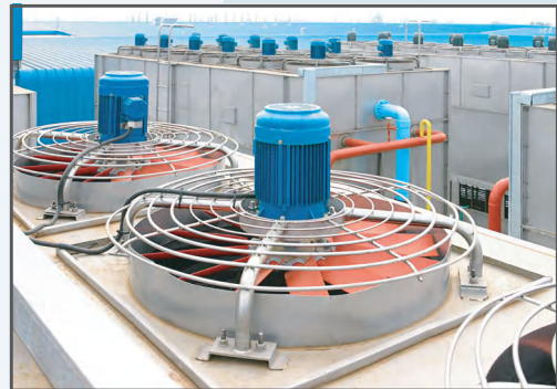
Fan and water pump
